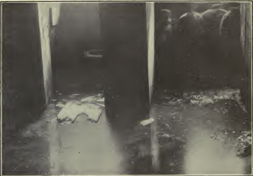
A flooded cellar toilet
